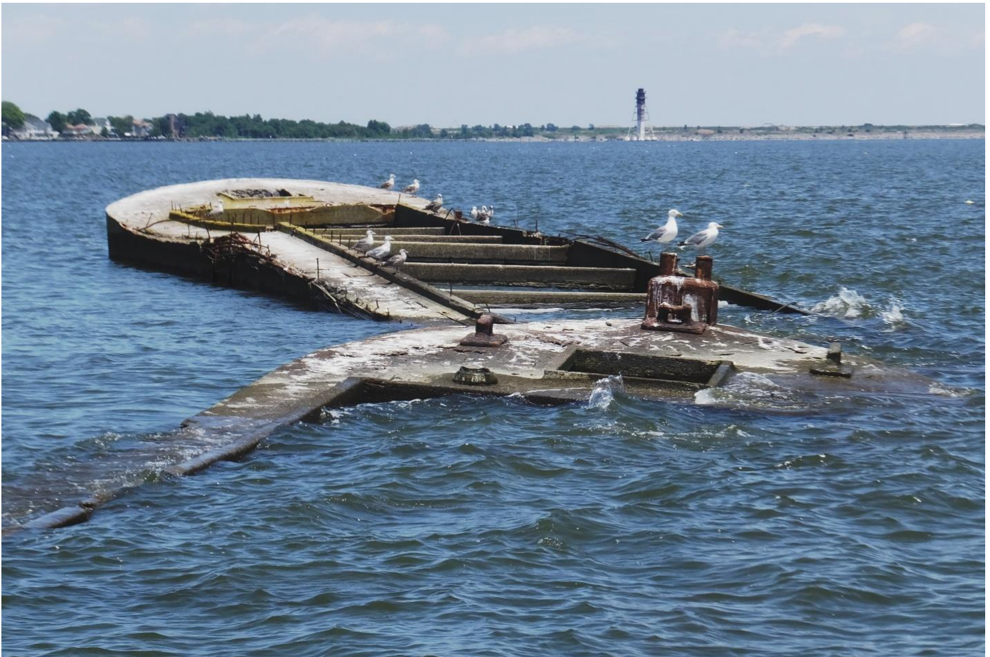
Figure 3: Concrete barges with the Craighill Channel Lower Rear Lighthouse in the background
